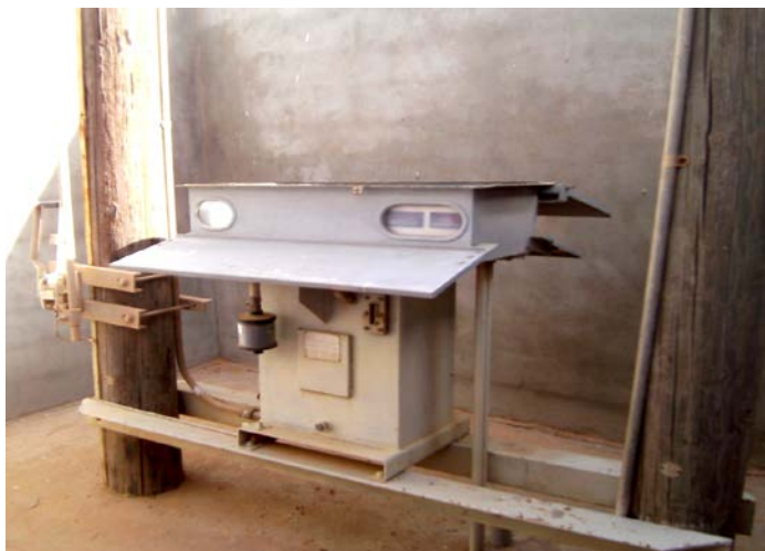
Figure 2.1- Rectifier at cathodic protection station no. 26.
