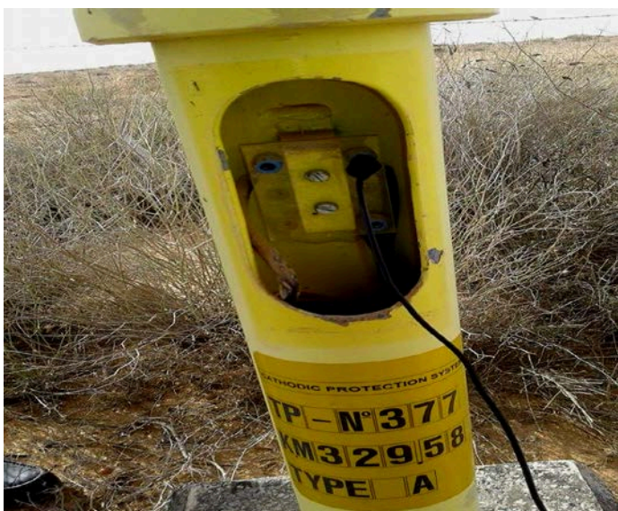
Figure 2.10 -Test post number 377 at 329.58 km from Brega city
