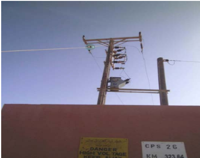
Figure 2.2- Step-down transformer at cathodic protection station 26.
